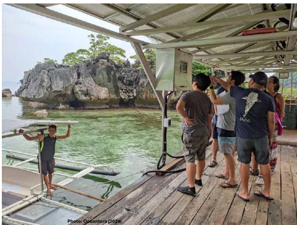
Figure 7. Charging station for Oceantera's e-boats.
